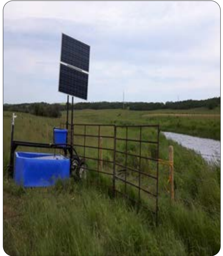
A solar powered remote water system and riparian area exclusion fence.
